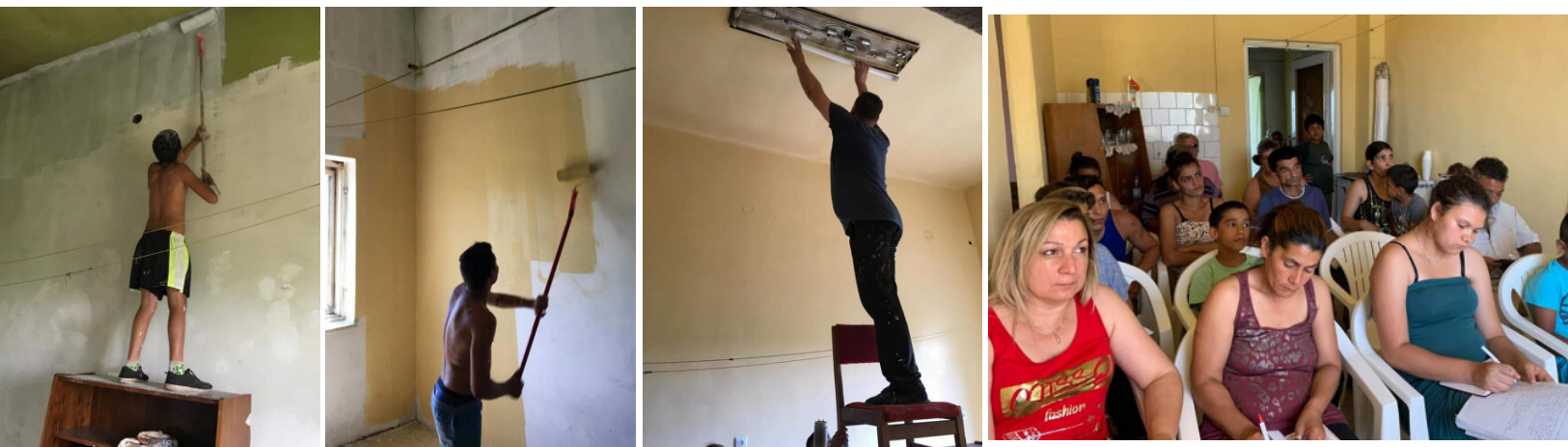
The pictures above (left to right) show the progression of the clean up and repair of the room where the Light to the Nations church meets in Bányzállás, Hungary, near the Southern border of Slovakia. Primer, then paint, and putting up a real light fixture and new chairs made the room unrecognizable from its former appearance. The people of Bányzállás, led by Pastor Istvan and Sylvia Sule did an amazing job cleaning, repairing and making a very nice place to have a church meeting as well as Light to the Nations Bible school. Thank you partners for making this possible. We are also thankful there were no injuries, even though safety precautions were not a high priority, as you can see.
